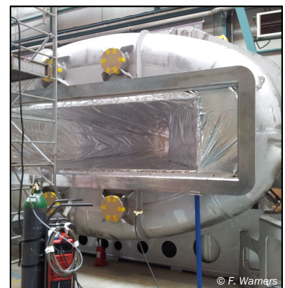
In the French Technology Research Center CEA Saclay the superconducting coils of GLAD were inserted into the cryostat, with which the magnet can be cooled down to 4.5 Kelvin
