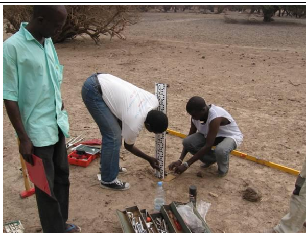
Photo 1 : Limnometric scale installation Niaka pond
