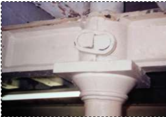
Fig 4 – Method of clamping cast iron beams to the supporting cast iron columns Source: Liverpool City Council
