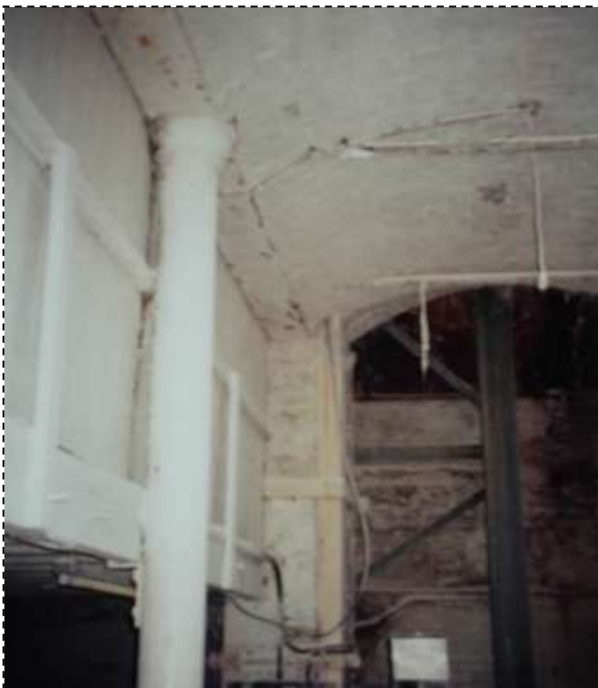
Fig 5 – Cast iron columns supporting with brick arch springing from the cast iron beams and wrought iron ties preventing spread. Source: Liverpool City Council
