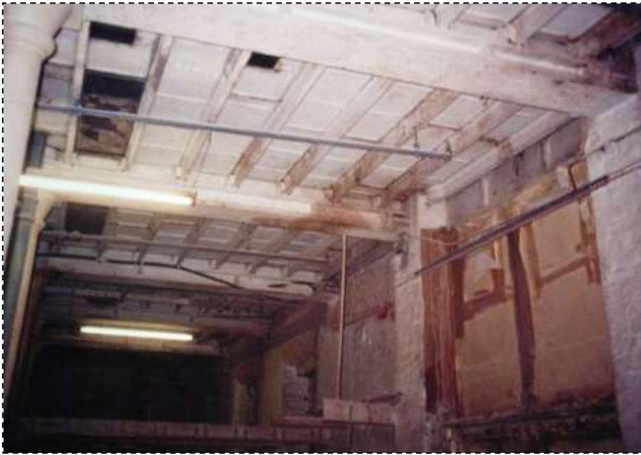
Fig 3 – Underside of iron plate floor on iron joists Source: Liverpool City Council
